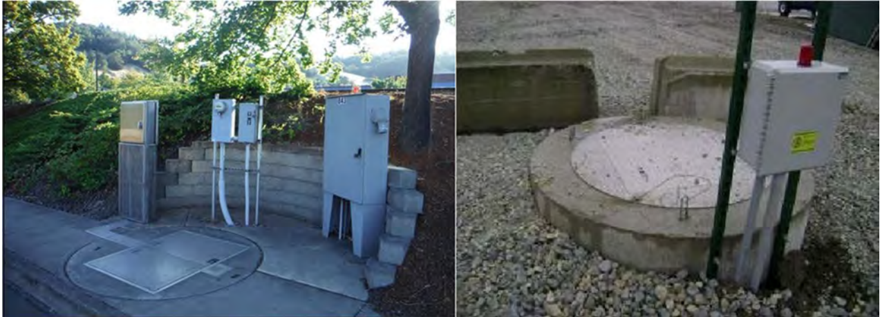
Figure 2-5. Examples of Below-grade Pump Stations (left: large, approximately 8 feet in diameter; right: small, approximately 3 feet in diameter)
